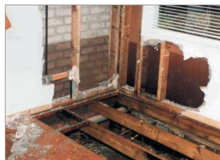
Fig. 4. Drying out a timber frame wall and floor structure after flooding (Courtesy of BRE)
