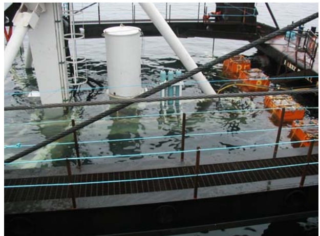
Figure 55: Ballast, pod and accumulators visible on recovery
