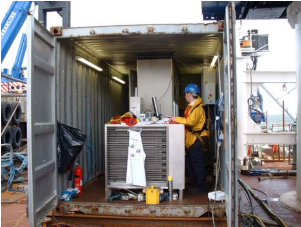
Figure 47: Working on the drive interfaces in the Control Cabin
