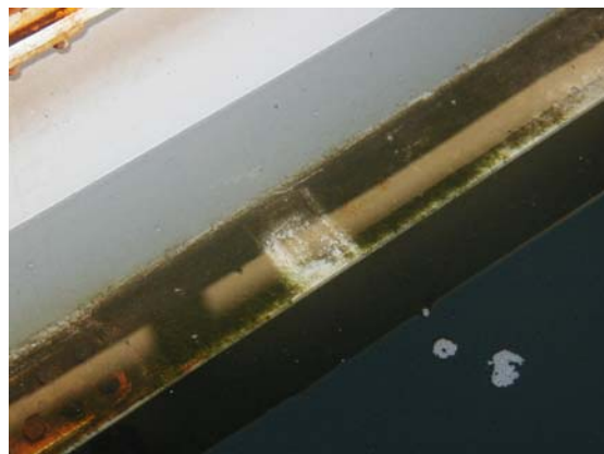
Figure 11: Minor further growth noted on recovery
