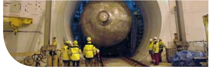
The first Steam Generator was successfully installed on November 17 in the Reactor Building.
