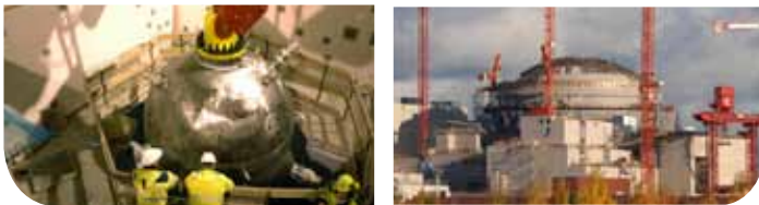
The pressurizer is more than 14m long and weighs more than 160 tons.
