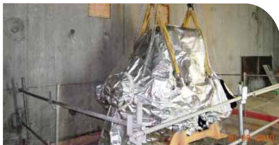
SIS pumps introduction, France
