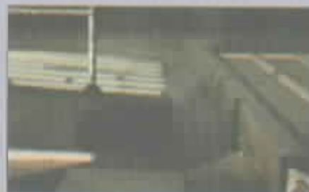
Air leakage through air duct and stairwell.
