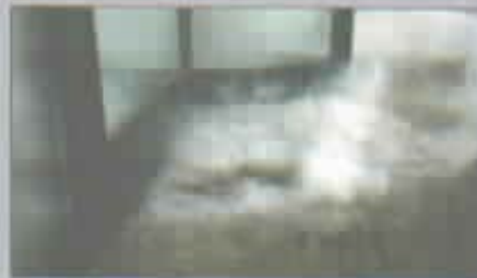
Air leaking through the seats of the revolving door serving the main entrance.
