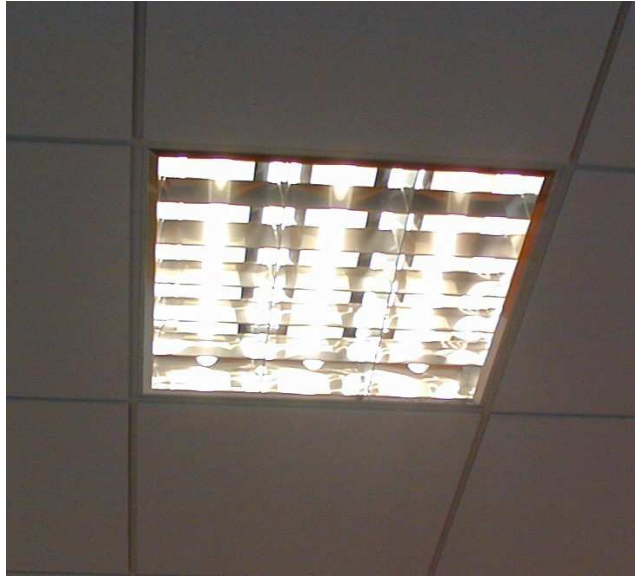
Fig. 16. Typical lighting fitting on both ground and first floors
