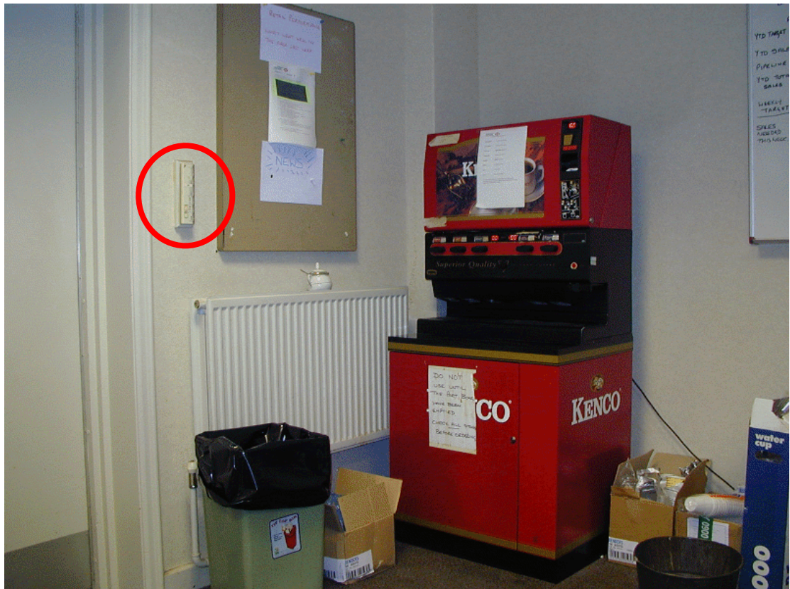
Fig. 50. The corner of the downstairs office. All heating is provided by panel radiators as shown with some having fins. All radiators are equipped with thermostatic valves although some need a little attention. The control for the air-conditioning is shown highlighted by the red circle. This is a confusing unit and few, if any, staff appear aware how to control it.
