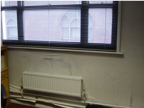
Fig. 36. Dampness on inside of building
