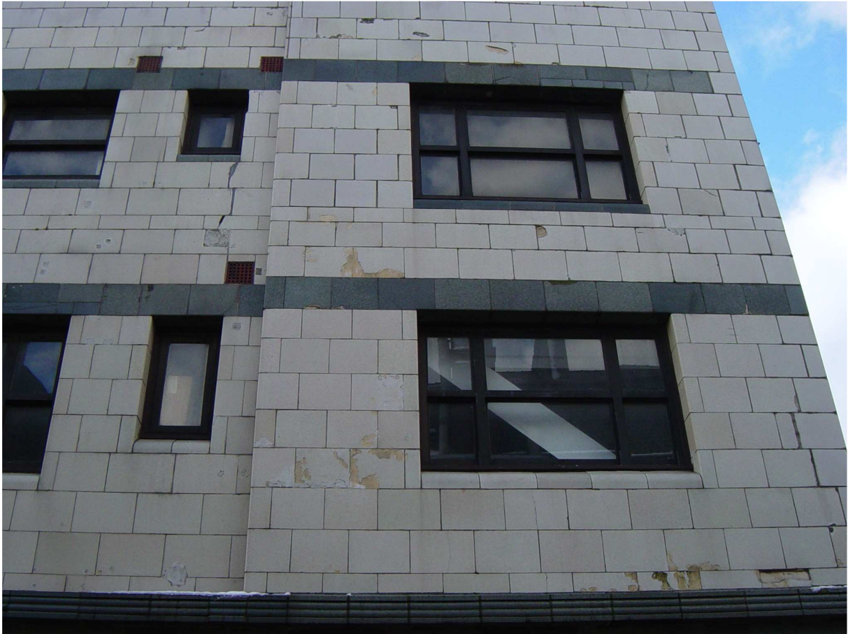
Fig. 35. View of the side of the building showing the problems with the tiles. It was reported that some had fallen off and been cemented back on.
