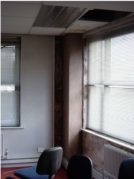
Fig. 37 Room now unusable
