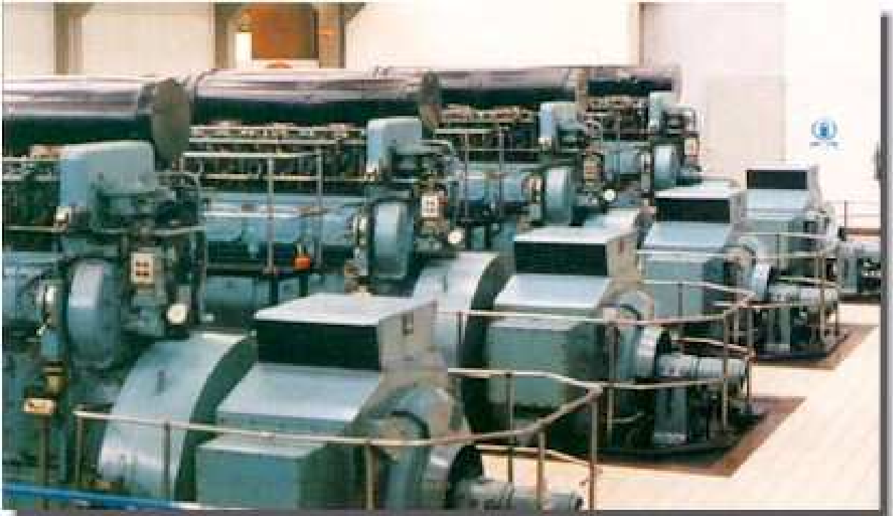
CHP Plant: Acknowledgement Gas Engineering Services Web Page
